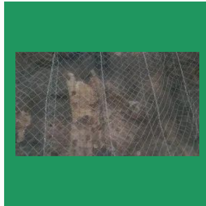
Rock Fall Netting
